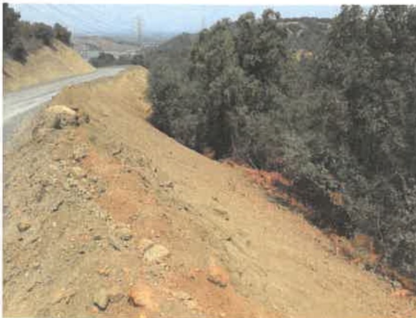
Figure 2: Observed Current Road Fill Profile
