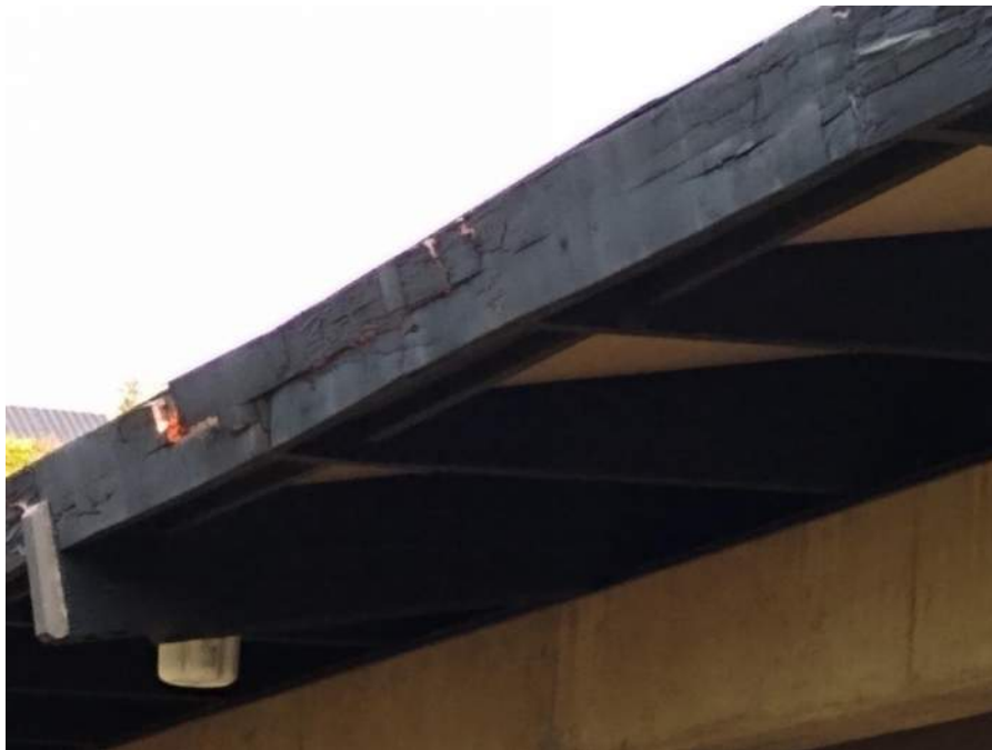
Photo 3 Damaged Veranda Fascia
