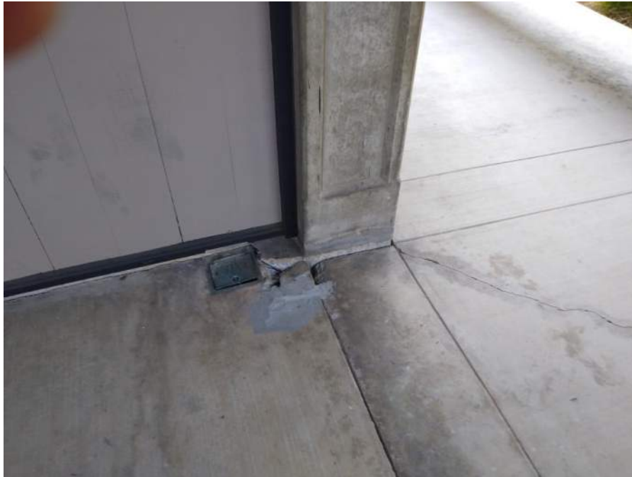
Photo 6 Veranda Damaged Slab on Grade
