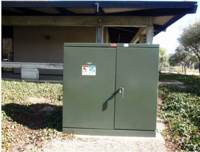
Figure 1E (PG&E Transformer)
