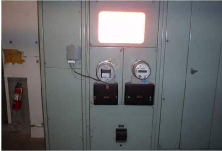
Figure 5F (Main Switchboard)
