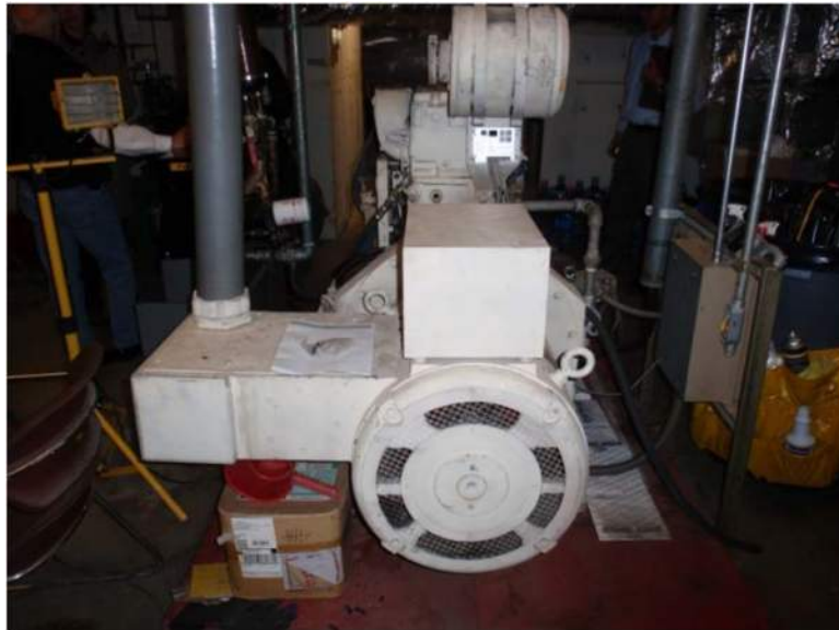
Figure 5G (Indoor Generator)
