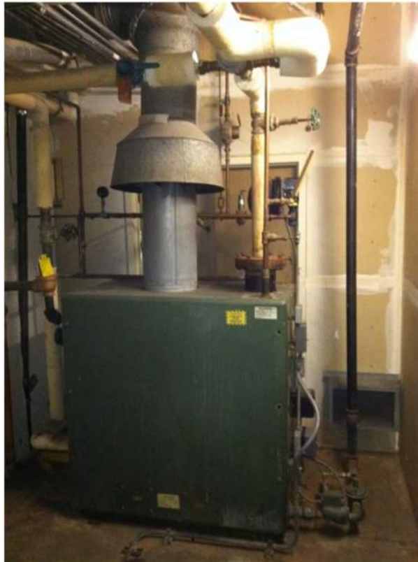
Figure 5C (Gas Fired Boiler)
