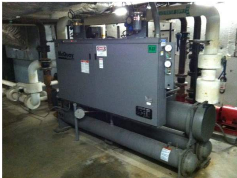
Figure 5B (Water-cooled 70 Ton Chiller)
