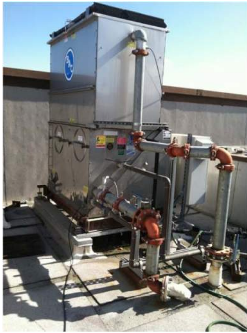
Figure 5A (Closed-Circuit 70 Ton Cooling Tower)
