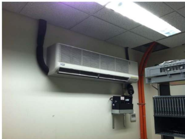
Figure 5D (Server room AC unit (1 of 2))
